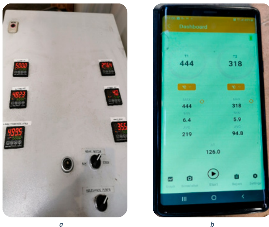
Fig. 4 Temperature monitoring during pyrolysis. a) Temperature control panel for the heating zones, reactor tube, condenser outlet and cooling water, and b) internal temperature monitoring during the pyrolysis process.
